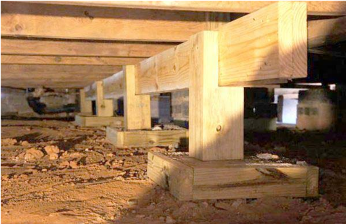
Wood beams were added to this house's foundation, which was initially poorly constructed.
