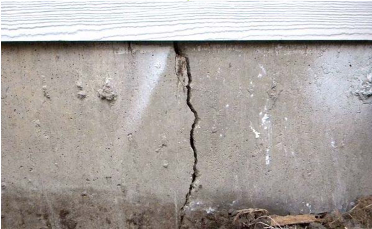
Drought is to blame for the crack in this house's foundation.
